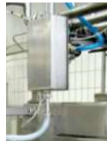
fig. 5: Separator installed at process sample line the outlet of the
